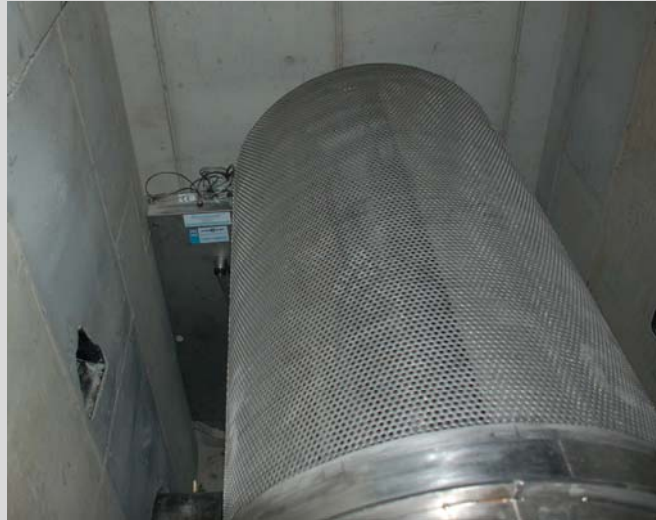
Hydroslide (lower left) and Cyclone (foreground) in the precast overflow chamber
