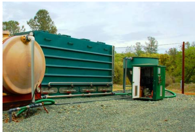
SAF at Yuba Co. with Septic tank in foreground and control kiosk and secondary clarifier in background.
